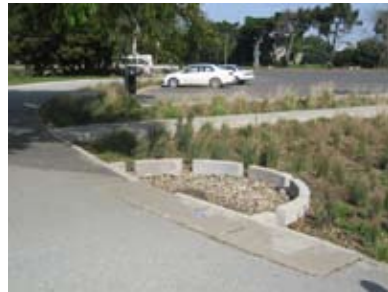
An infiltration basin at Lake Merced
