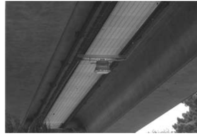
Inset lighting on the Ohlone Greenway
